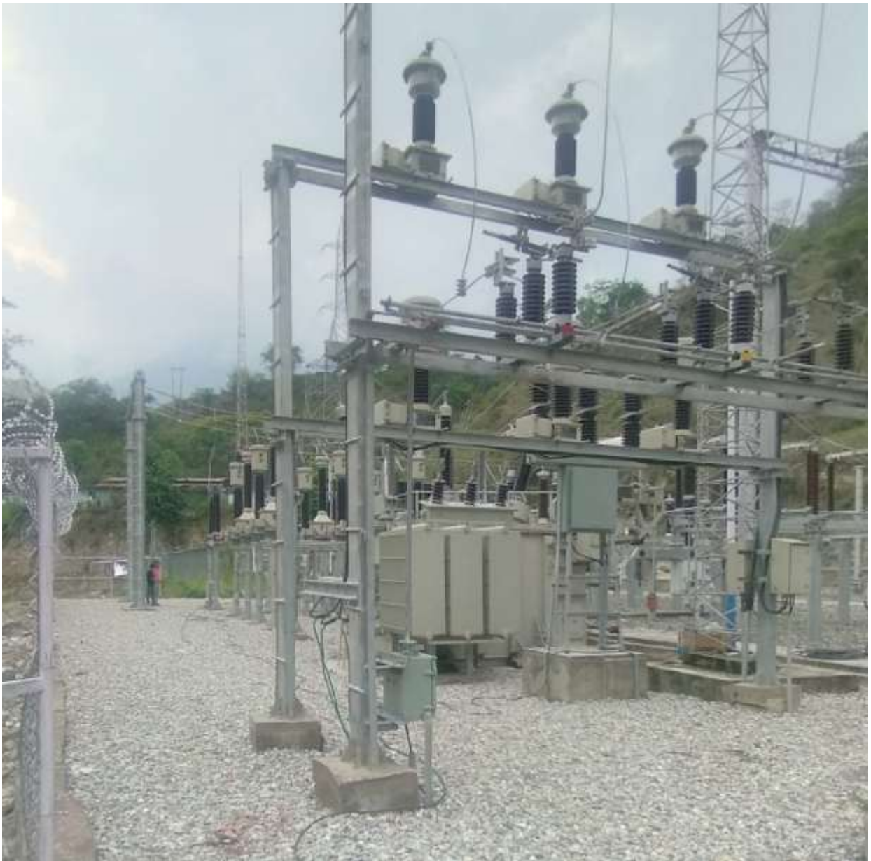
Photo 8-5: Interconnection Substation of Hidi HPP at Nyadi HPP Switchyard
