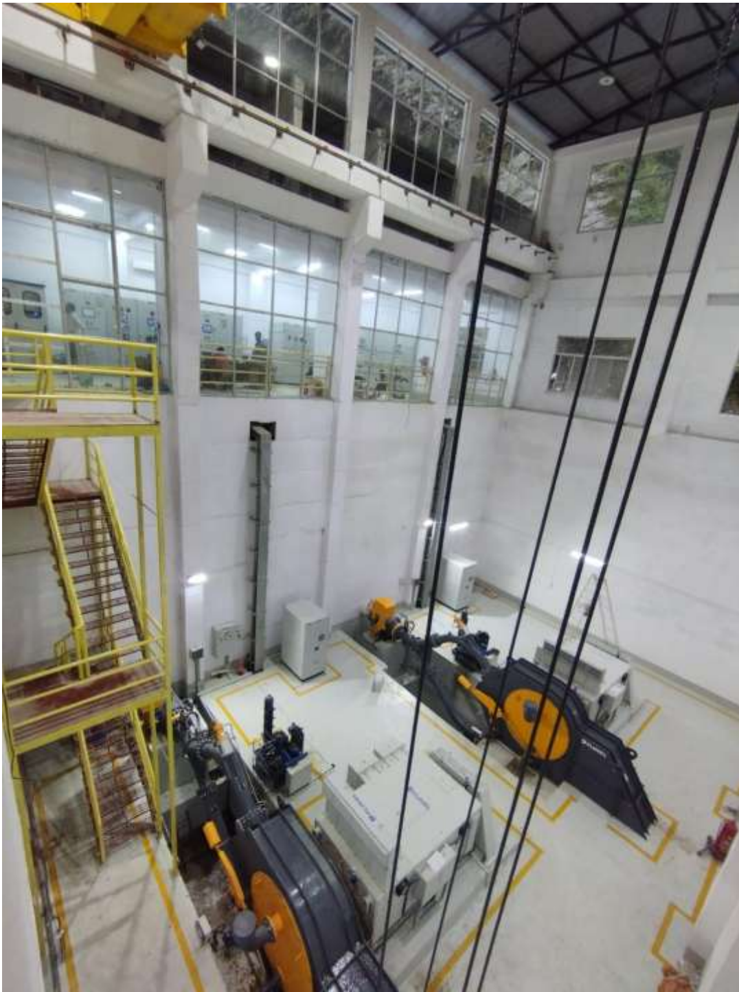
Photo 8-3 EM equipment at Powerhouse
