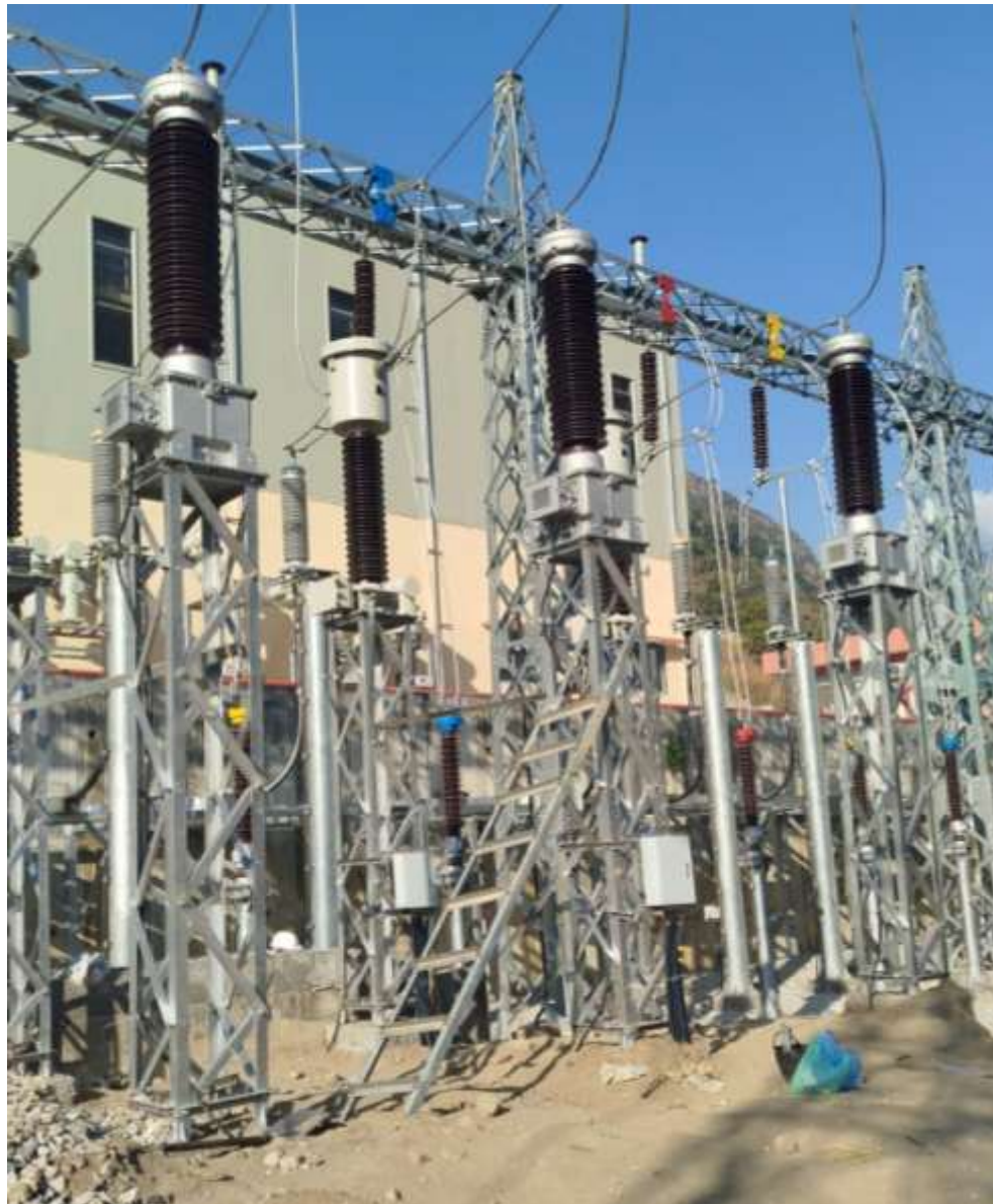
Photo 8-6 Support structure for CT , VT at Khudi Substation
