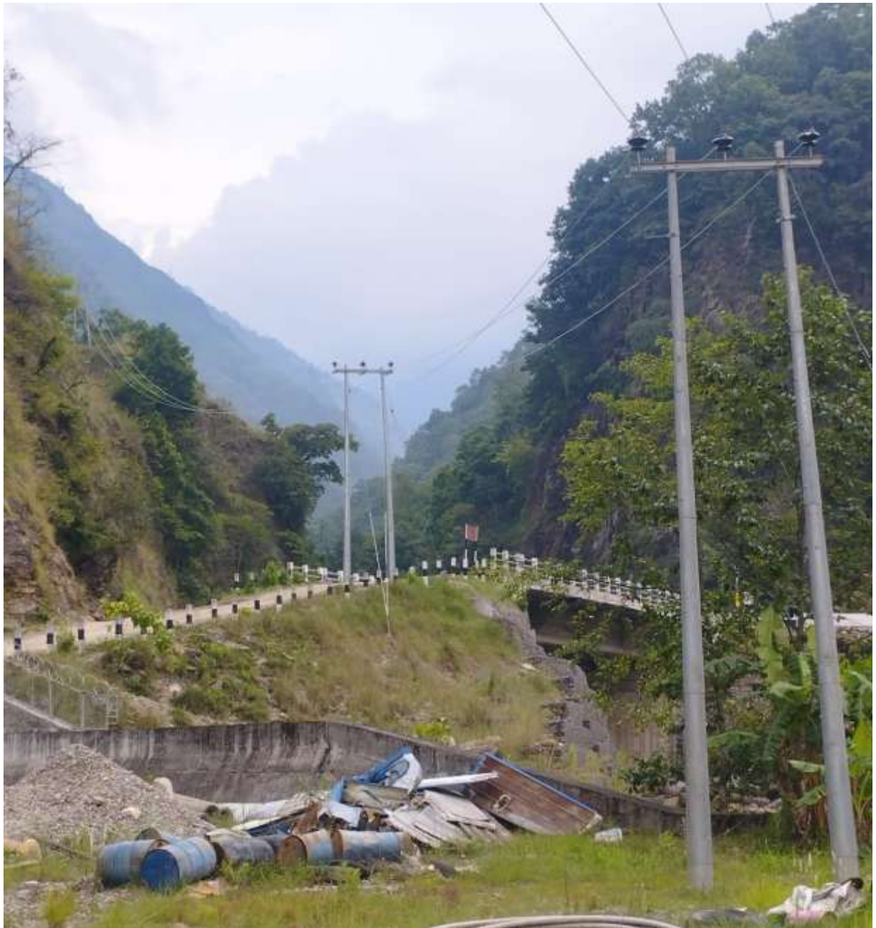
Photo 8-4 33 kV Transmission Line of Hidi Khola HPP
